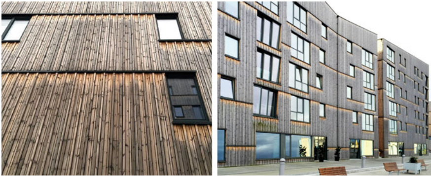
Fig. 5.3 Weathered building in Stavanger, Norway. Image courtesy of Lone Ross Gobakken, NIBIO
