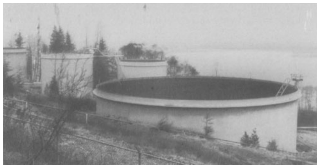
Plate 2.1. Floating roof petroleum storage tank for the control of hydrocarbon vapour loss. Roof is sunk below the rim of this partially empty tank, shown by inclined service walkway.
