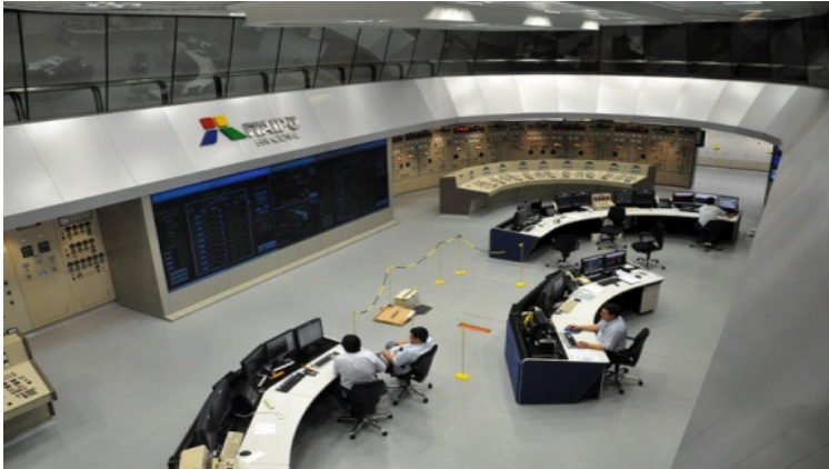
Fig. 2. Typical Electric Power Control and Operation Center
