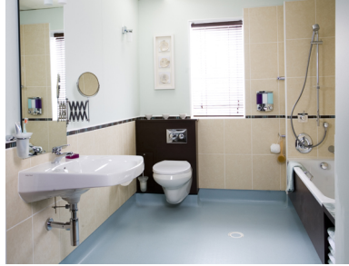
Fig. 7. Slip-resistant flooring and contrasting colours between the floor, walls and sanitary ware for additional safety and user orientation
