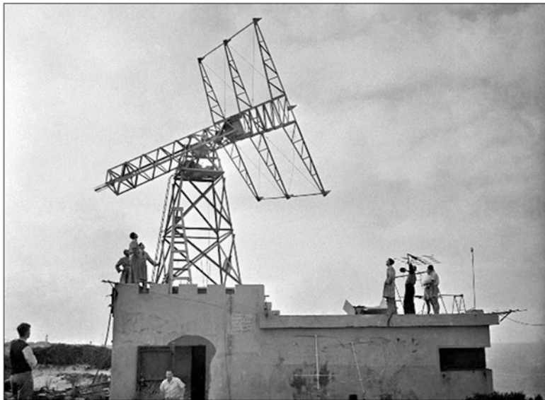
Fig. 2.17 The 9-Yagi array under construction early in 1949, with two of the Yagis leaning against the blockhouse. The array with its equatorial mount was used to carry out the first survey of the southern sky (courtesy: Stanley family)
