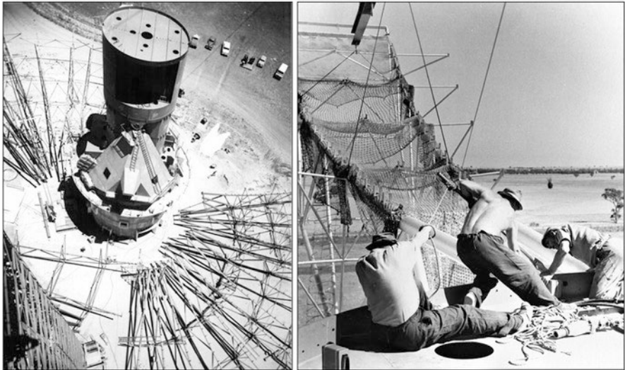
Fig. 5.3 The construction of the Parkes dish during 1959–1961 was carried out by the German steelmaker MAN. Most of the components of the telescope were cast at the MAN plant near Frankfurt and then shipped to Sydney (courtesy: CRAIA)
