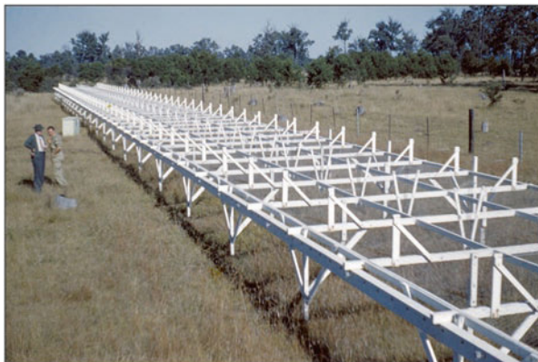
Fig. 4.26 The 50-dipole N–S array under construction at the Wallacia field station (courtesy: CRAIA)
