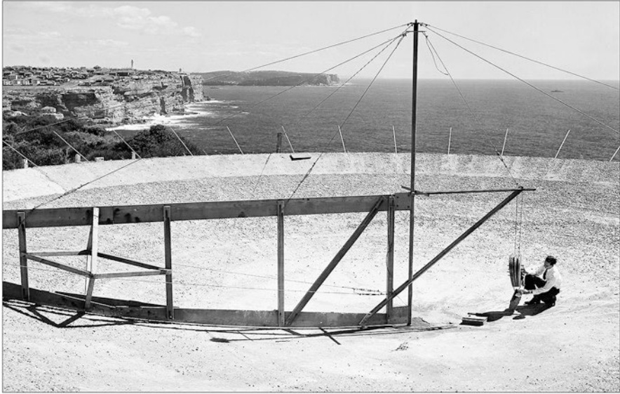
Fig. 2.23 Upgrading the hole-in-the-ground in February 1953 – a concrete surface was added and the diameter extended from 22 to 24.4 m. The rotating parabolic template was used to position formwork for the concrete and also to finish the surface (courtesy: CRAIA)
