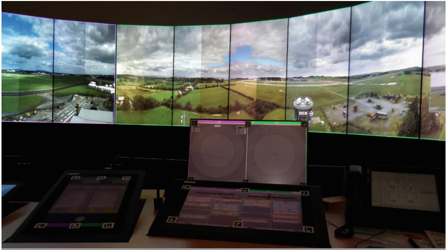
Fig. 1. The Module of multiple remote tower control system comprised by Electronic Flight Strip (EFS), Out of the Window (OTW), Radar Data Processing (RDP), Information Data Processing (IDP) and Voice Communication System
