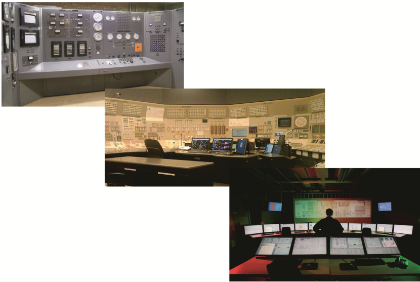
Fig. 1. Three generations of nuclear power plant control rooms (top to bottom: EBR-1, the first nuclear power plant with an all analog control room; recently decommissioned San Onofre Nuclear Generating Station, with a hybrid analog-digital control room; HAMMLab at Halden Reactor Project, a fully digital advanced control room concept).
