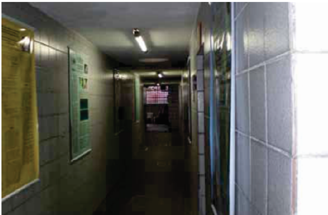
Fig. 3. The lighting is precarious in the corridors
