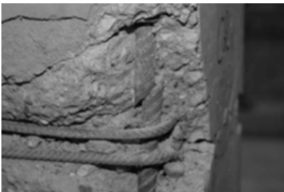
Fig. 4.15 The mistake in the construction of the hoops (and the resulting impaired confinement) led to heavy damage of the precast column in the PRECAST full-scale test
