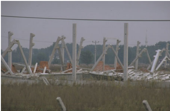
Fig. 4.10 This collapsed precast structure illustrates the importance of ties in precast buildings
