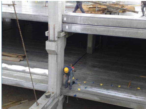
Fig. 4.5 Beam-to-column dowel connection is clearly seen in the upper floor. In the lower floor the beam has been already installed and the steel sockets will be grouted
