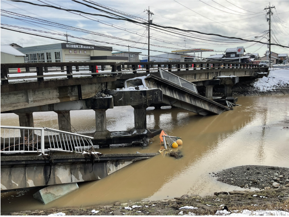
Fig. 2. Sidewalk collapse of Ukai Bridge subjected to ground motion and/or tsunami caused by 2024 Noto-Hanto earthquake. Note that the picture was taken by the second author.
