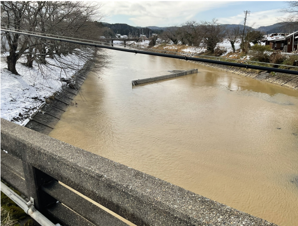
Fig. 3. Washout of Ukai Bridge sidewalk due to tsunami caused by the 2024 Noto-Hanto earthquake. Note that the picture was taken by the second author.
