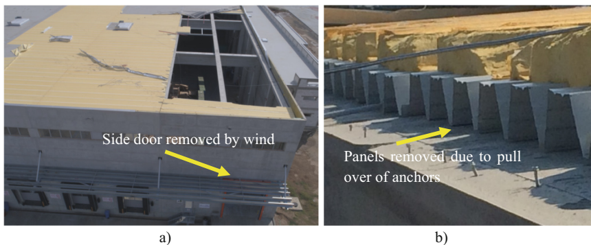
Fig. 15. Roof (and side door) destroyed by wind: a) aerial view with the damaged roof; b) detail with end support fasteners in the affected roof area.
