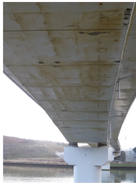
Fig. 5. Bridge redeterioration due to chloride attack after repair near Noto Peninsula (Note that the picture was taken in 2017 by the second author)
