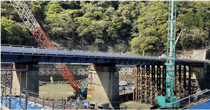
Fig. 9. Washout of superstructure due to the 2020 Kyushu flood and reconstruction of temporary bridge using the survived bridge piers in Kuma River. Note that the picture was taken by the second author.
