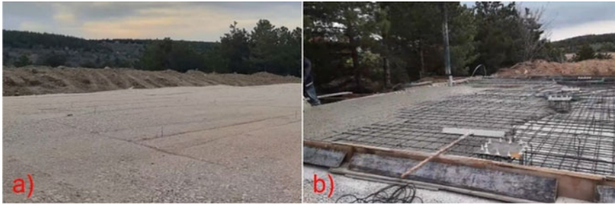
Fig. 14.5 Construction of the mat foundation, a laying of gravel; b building of the foundation
