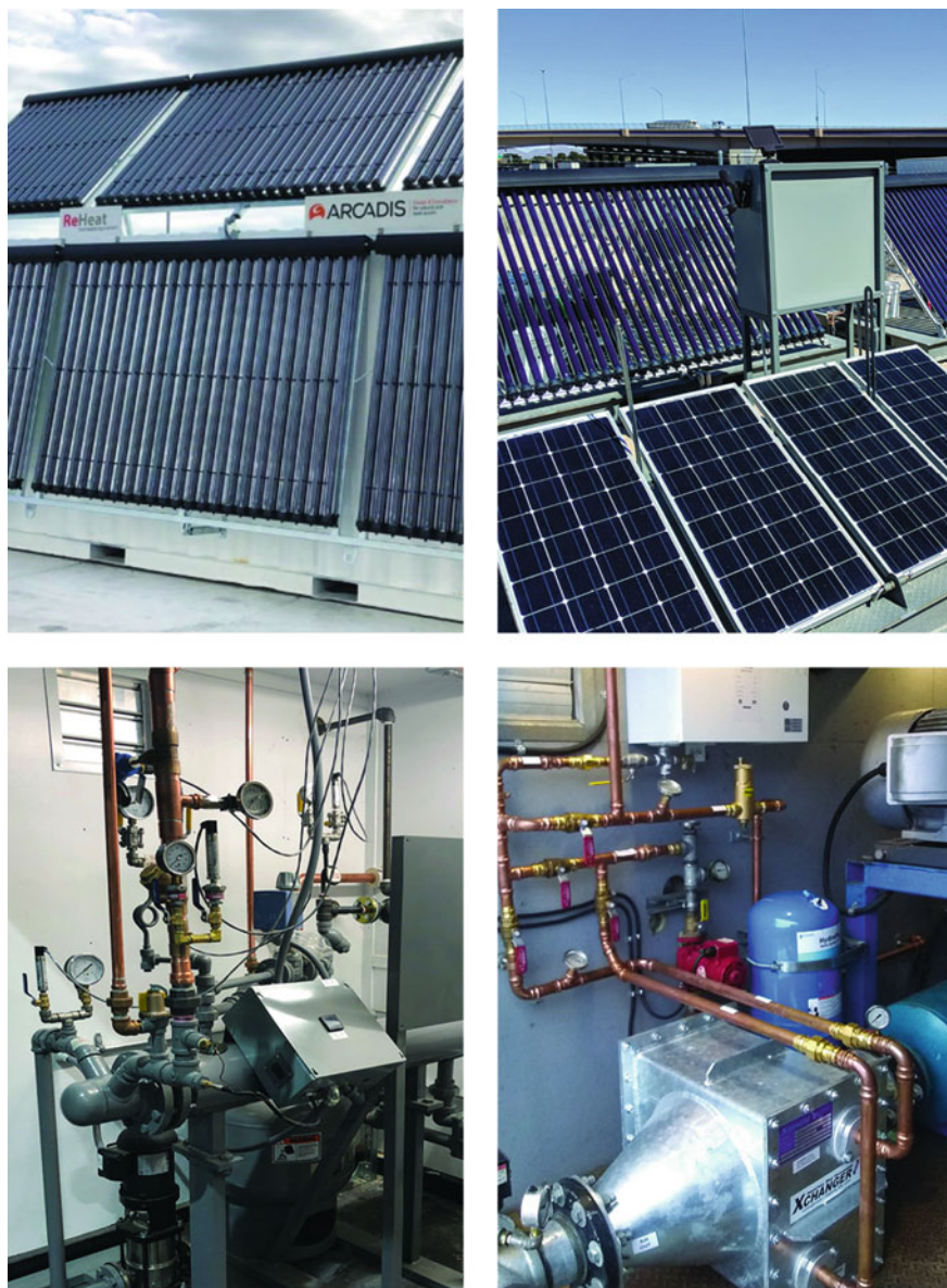
Fig. 18.8 TISR infrastructure for solar energy (solar collectors) and waste heating (blower heat exchanger) applications
