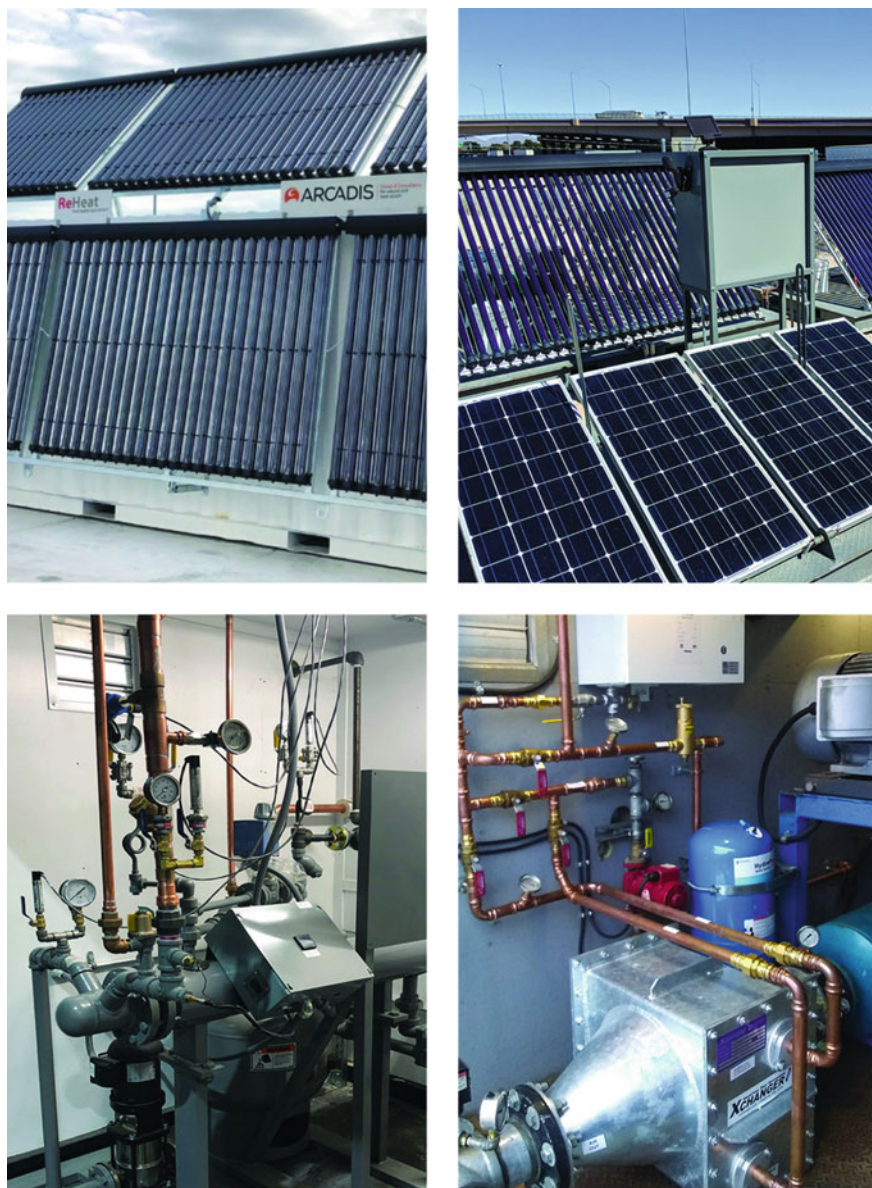
Fig. 18.8 TISR infrastructure for solar energy (solar collectors) and waste heating (blower heat exchanger) applications
