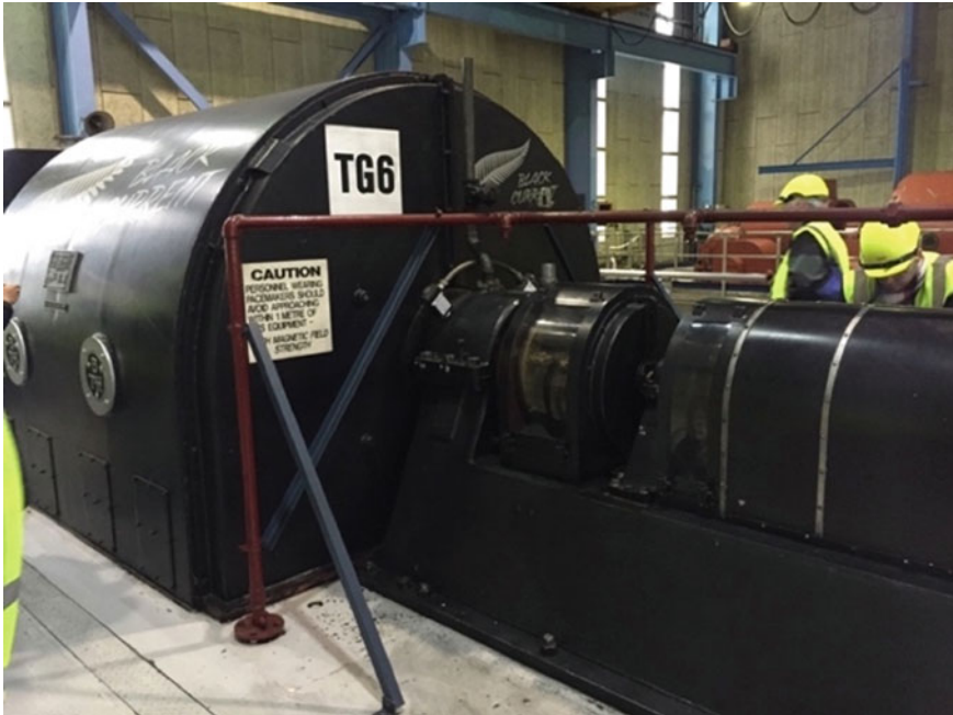
Fig. 19.1 The Black Current Generator currently in the Ohaaki Geothermal Power Station, New Zealand showcases the robustness of the technology where many early generators from the 1960s are still operable today (©Klaus Regenauer-Lieb)
