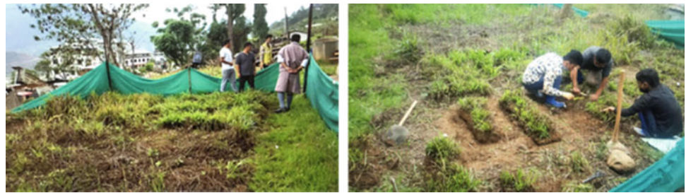
Fig. 9 Plant bed for Type C vegetation works. The grass to transplant is first removed in stripes from the plant bed
