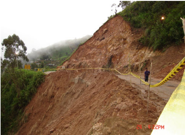
Fig. 10 Upper and lower slope de-stabilization after construction of a road in mountain environment
