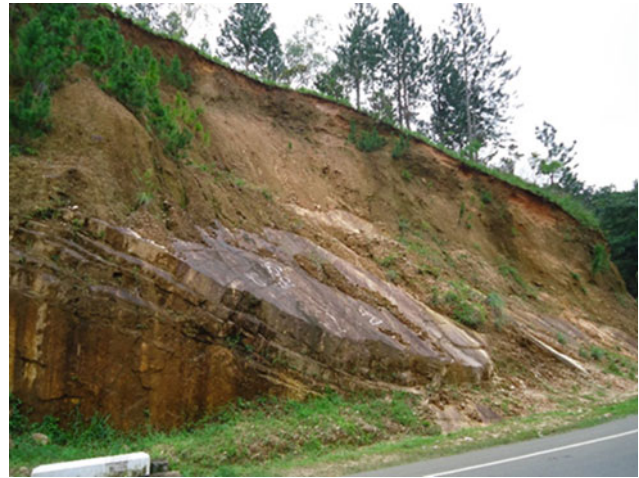
Fig. 12 Failure observation of a road side slope cut section which was constructed at 0.5 to 3.5 m high without any retaining structures
