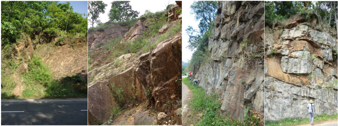
Fig. 13 Example of rock formed failures along the road side slope. Wedge failure, translational slides and falling rocks are very much significant along the road sides. High hazard potential zone can be observed due to foliated and jointed rock formations
