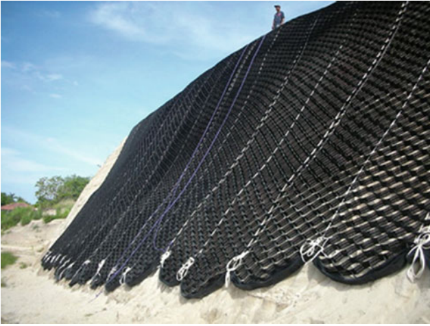
Fig. A.1 Geosynthetics used to stabilize a slope using soil in-fill and seeding for plants
