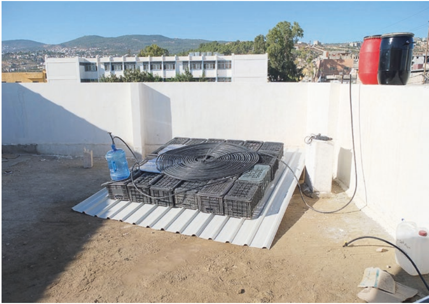
Fig. 1 A simple system for heating water and insulating the zinc roofs developed specifically for and with refugees in Jerash camp (Source: Students of TU Berlin, 2016)
