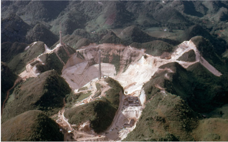
Fig. 38.5 Aerial view of the Arecibo construction site, September 1961. Joe and Lenore Pawsey Family Collection
