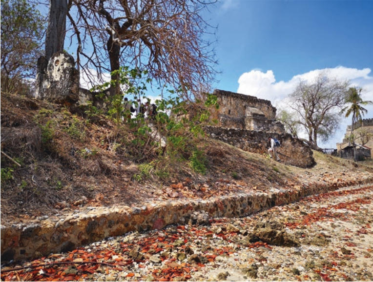
Fig. 18.2 Gabion wall below the Malindi Mosque at Kilwa Kisiwani. ( Note: Photograph by William Megarry, 2018)
