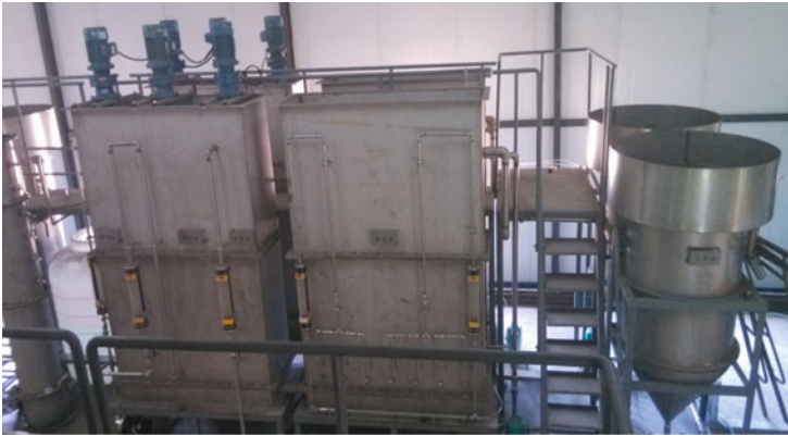
Fig. 4.6 Chinese modified AAO pilot plant for combined treatment of municipal and pharmaceutical wastewater in Shenyang (FiW)
