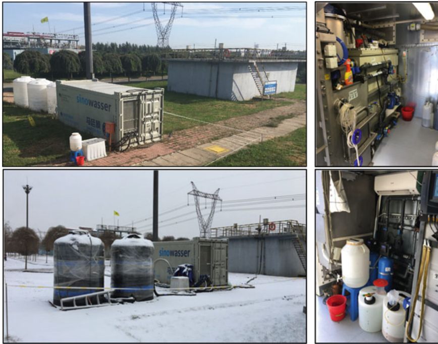
Fig. 4.11 SINOWATER experimental plant in summer (top), winter (bottom left) and interior views (right) (FiW)
