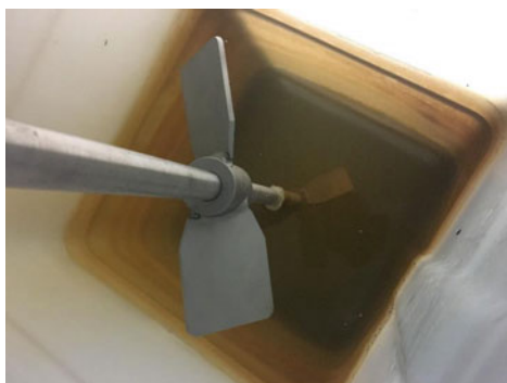
Annex 4-4: flocculation tank (inside) and agitator (FiW)
