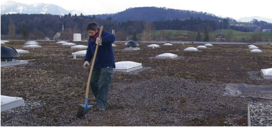
Fig. 2.4 Setup of uneven topography on a green roof. In order to enhance plant and animal (e.g. arthropod) biomass, the environmental conditions of some of the selected roofs were improved by adding a layer 8–16 mm-thick of expanded slate on the pre-existing substrate (30 mm-thick layer of pumice lava and clay) hosting sparse ‘moss and Sedum spp.’ vegetation. (Photo credit: Nathalie Baumann 2009)
