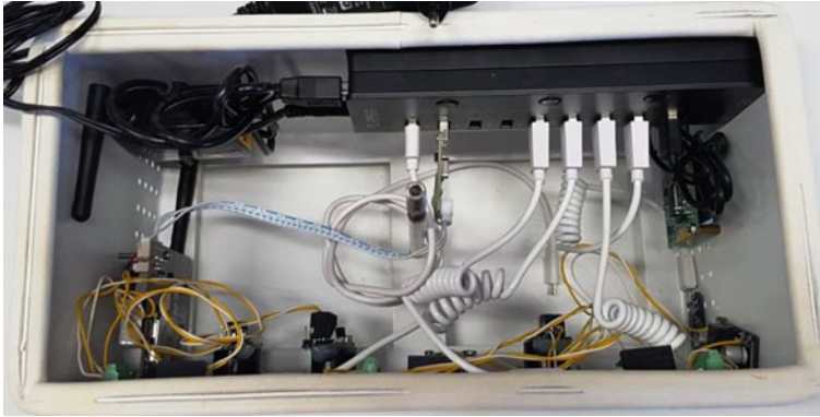
Fig. 11 Sensors, smart router and connectors
