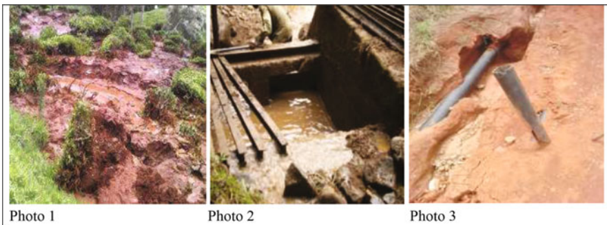
Plate 1 Impacts of heavy downpour on the water system
