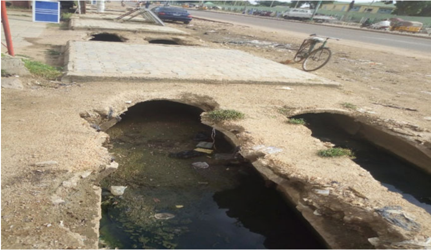
Fig. 7 Poor drainage filled up with silt, obstructing the free flow of storm water along Dala Orthopaedics Gwammaja. (Source: Field Survey 2019)
