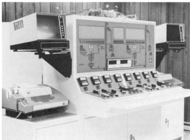
Fig. 5. Feed mill computer allows operator to follow major ingredients from bins into scale, then mixers, where liquid and bag dump ingredients are added. The panel has controls for two independent batching systems. (Boone Valley Co-op Processing Association, Eagle Grove, Iowa)
