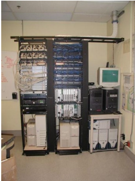
Figure 1-5. RDCC private data center (courtesy of Microsoft)
