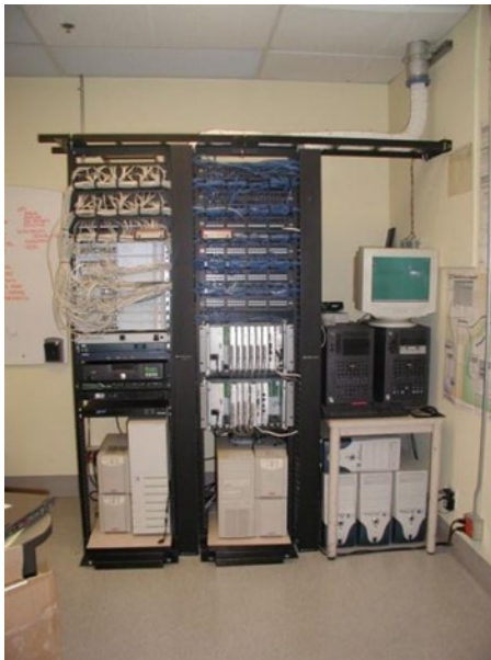
Figure 1-5. RDCC private data center (courtesy of Microsoft)
