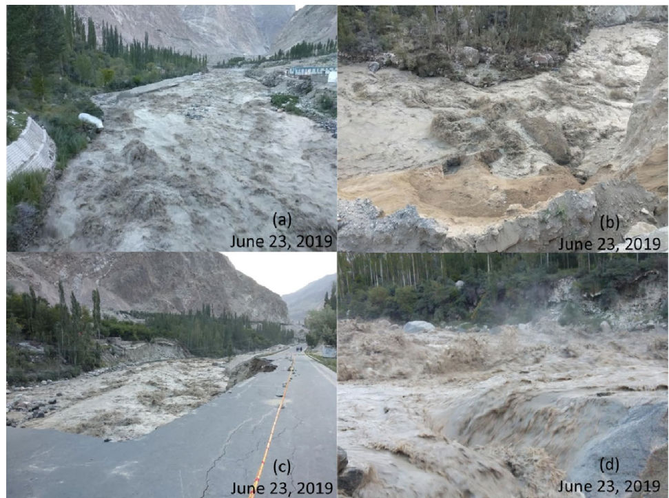
Fig. 12 Pictures of damages to downstream infrastructure taken on June 23, 2019, due to sudden release of flush-muddy seepage-water discharged from the ice-dammed Shishper glacier lake. The recently made mitigation walls on both sides of the gorge to reduce the impact of ice-dammed glacier flood (a) outburst flood hitting the Karakoram Highway (connecting Pakistan with China) (b, c) damages done to forest on both sides of gorge (d)
