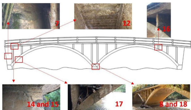
Fig. 8 Elevation view of the bridge with defects obtained by traditional inspection
