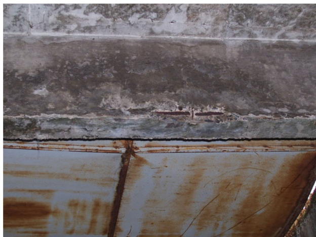
Fig. 5 Rebar exposes on the beam
