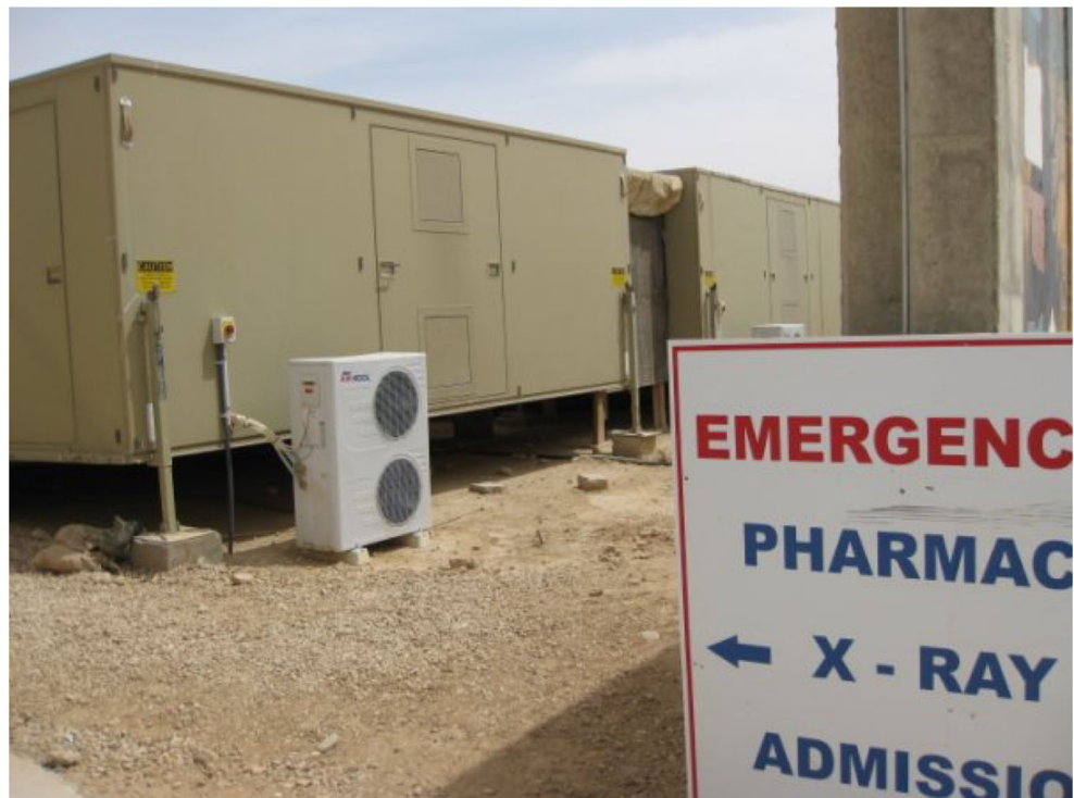
Fig. 1 International organization for Standardization Shelter (ISO-Shelter) used to house radiology equipment as part of a Combat Support Hospital (CSH)
