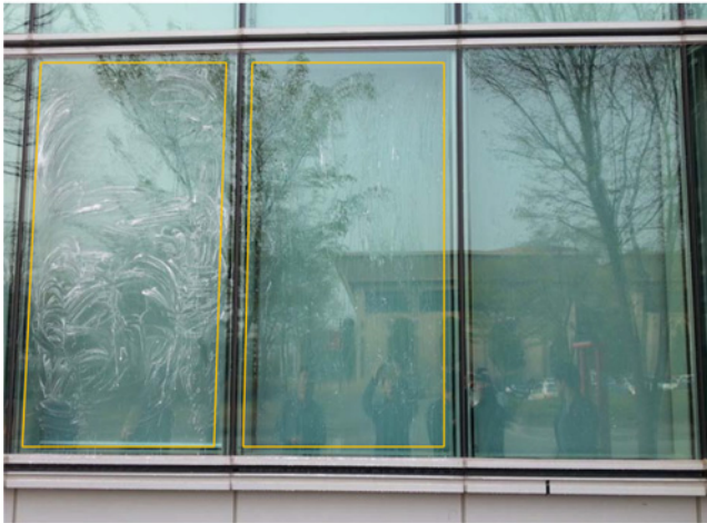
(a) Before cleaning
