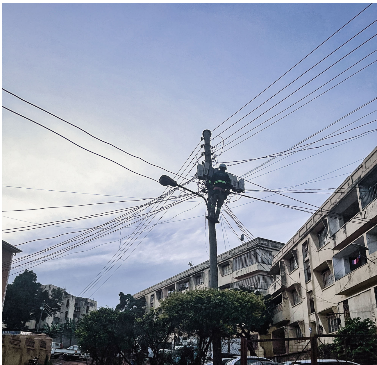
Fig. 3 An electricity service worker fixing a frequent power outage due to overcrowding of electricity wires in Kampala, Uganda
