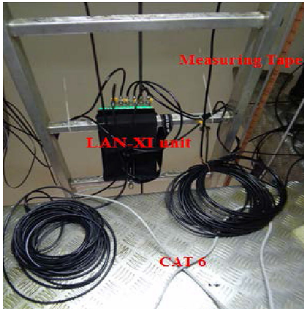
Fig. 8 LAN-XI unit fixed at the ladder
