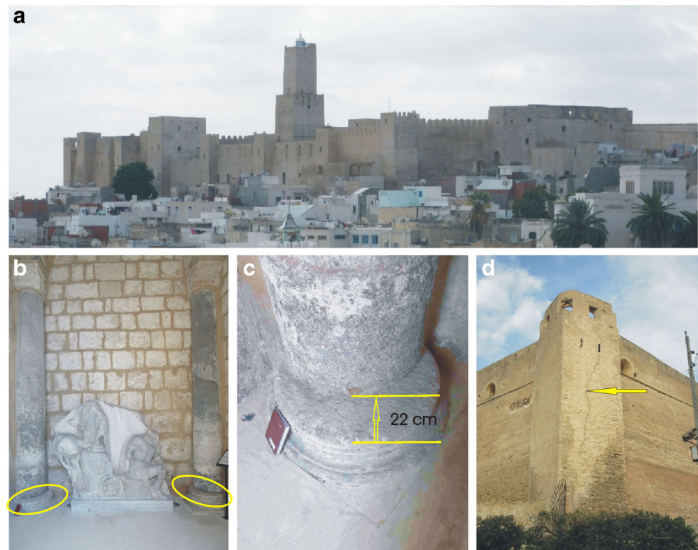
Fig. 5 Evidence for damaging earthquake affecting the kasbah in Sousse. a View of the huge fortress from northeast. #5857. b Both marble columns on the right and left are shifted on their respective plinths (encircled). #5926. I = IX. c Figure NW column at the kasbah museum entrance, shifted on the plinth by 22 cm in northwestern direction. #5928. I = IX. d Tower on the southwest corner is fractured vertically (arrow) (see also Bahrouni, 2020a: Fig. 7c). #5915. EMS98 intensity is assigned after Rodriguez-Pascua et al. (2013). 35° 49' 22" N, 10° 38' 09" E
