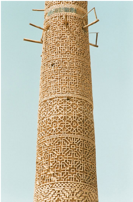
Fig. 29 The top portion of the Damghan minaret with four tiers of tetragonal rib patterns, all with the plane group p4mm . Patterns from the bottom: (1) Diagonally oriented unit cell with small squares and void crosses, respectively, on two sets of fourfold axes. (2) Eightfold stars and octagons define unit cell vertices and regular crosses are in the center of the cell. Oval polygons interconnect the octagons in this Islamic pattern repeatedly used at different monuments. (3) A very large diagonally poised unit cell with empty small squares in the corners and a complex cross-like arrangement of small squares in the center. (4) Pattern with a small unit cell and tighter line overlap; small squares and empty crosses mark the fourfold rotation axes
