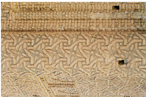
Fig. 8 A deceptively curvilinear pattern composed of straight brick segments. Symmetry p4 with fourfold rotation axes on the ‘flowers’ and on squares. A buttress of the W tower
