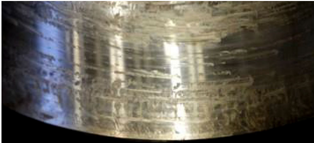
Fig. 9 Main bearing seat with inner ring creep damage observed in the project “BeBen XXL”
