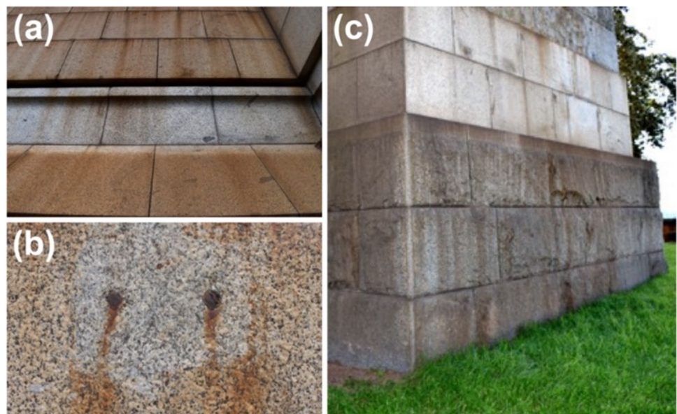
Fig. 2 a View of the side of the abutment tower, Western face, directly under the railway—rust stains, b close up on rusty stain formed around nails. c Environmental soiling and rust on the base of a Sydney Harbour Bridge pylon supporting the approach spans, facing South
