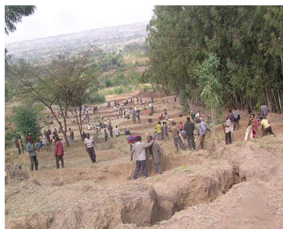
Figure 2 Public campaign workers building soil and water conservation measures in Hanja Chafa kebele, Chafa micro-watershed.
