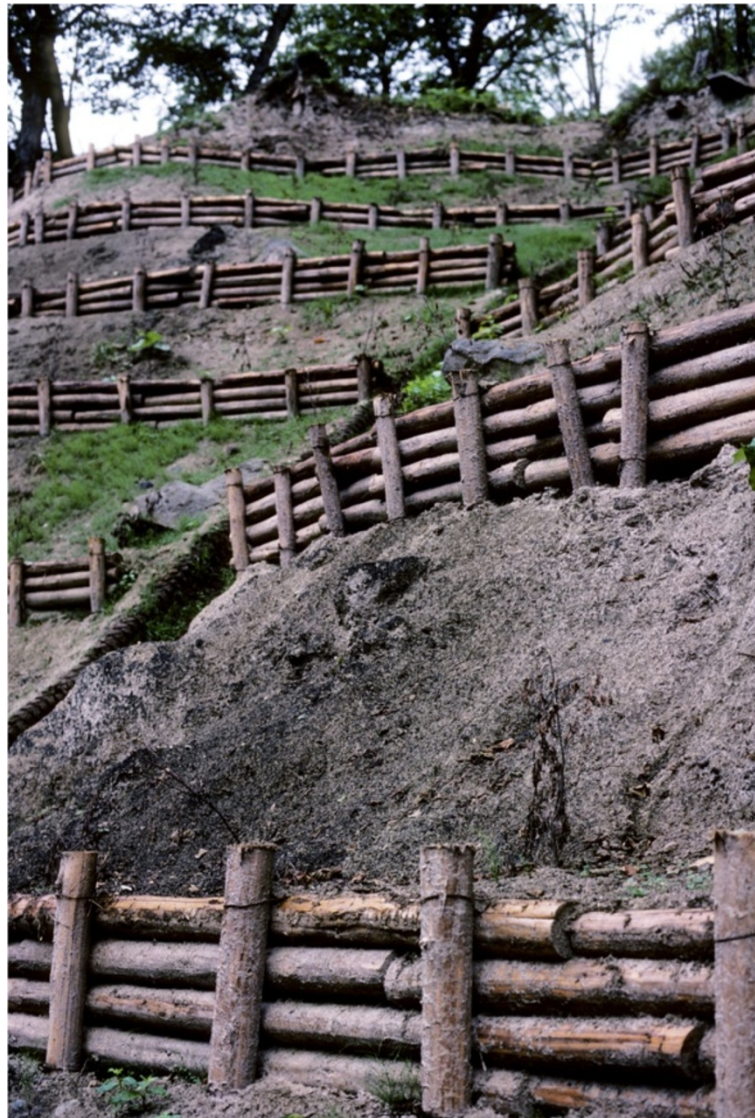
Figure 5 Example of slope stabilization. Timber retaining walls used to stabilize a steep slope in a volcanic area in Japan (USGS photo by TCP).
