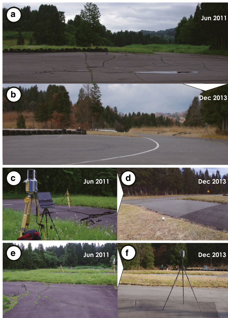
Fig. 2 Photographs of the site. a, c, e The open cracks on the surface pavement formed by the 2011 earthquake. b, d, f The repaired pavement. Photograph locations are shown in Fig. 1c
