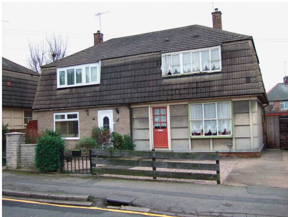
Figure 3: Different evolution of non-traditionally constructed semi-detached houses. The house still in its original form (right) requires significant refurbishment.
