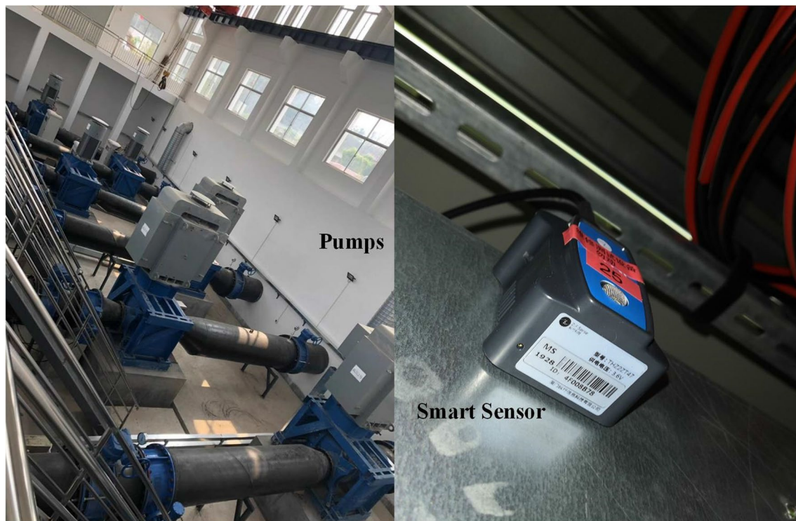
Fig. 5 Pumps (left) and smart sensor (right) in the water station
