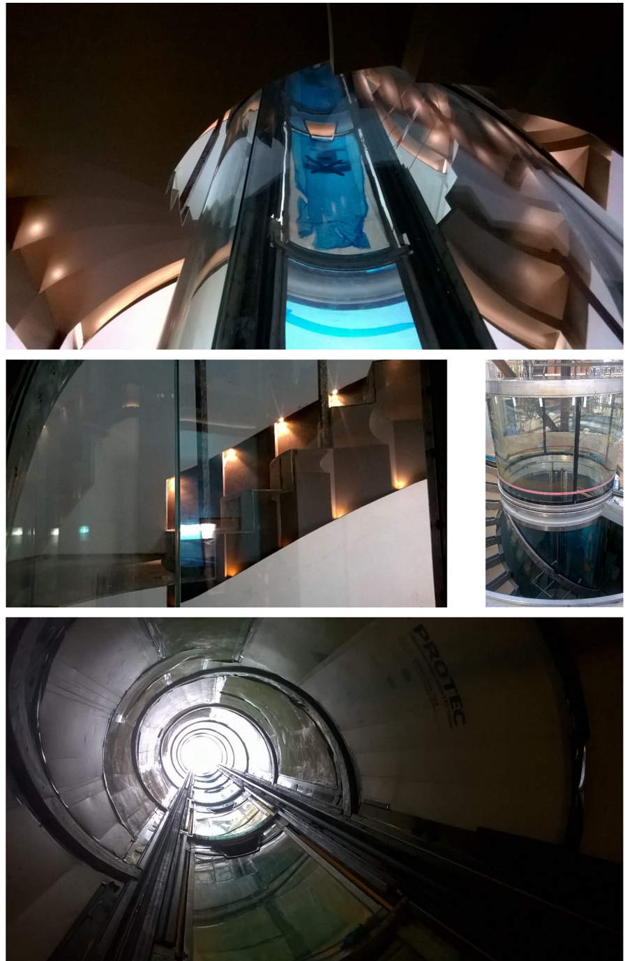
Fig. 15 View of the segment, across and top hat. View up completed shaft
