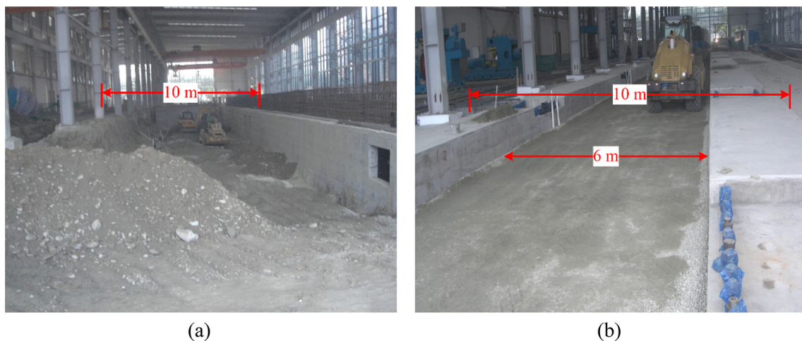
Fig. 6 Construction of the subgrade in the platform: a earthwork excavation; b compaction
