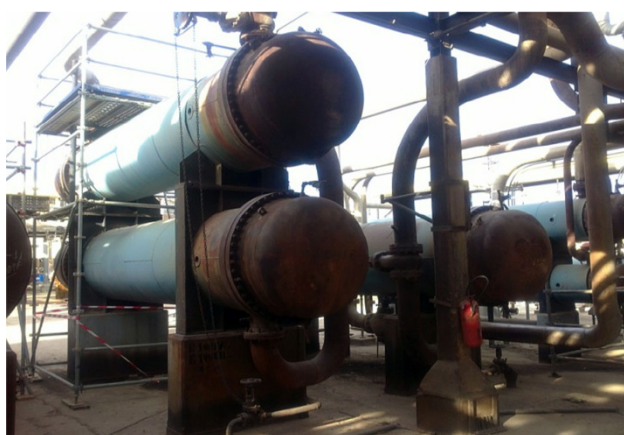
Fig. 4 Picture of the E101 CBA heat exchanger
