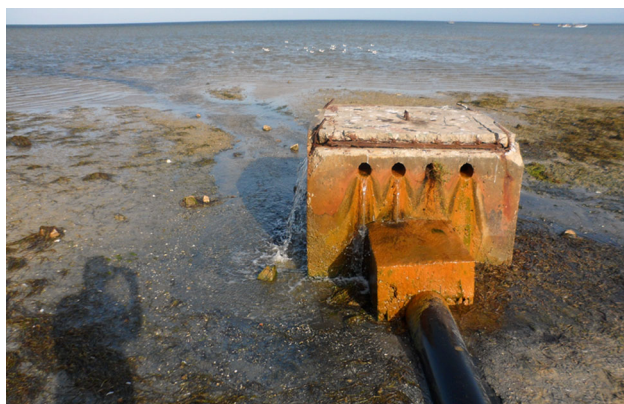
Fig. 3 Treated water coming from Sewage Unit and rejected in the sea
