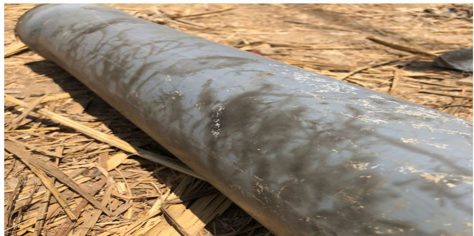
Fig. 11 The dark random streams on the outer surface of the aged uPVC pipes
