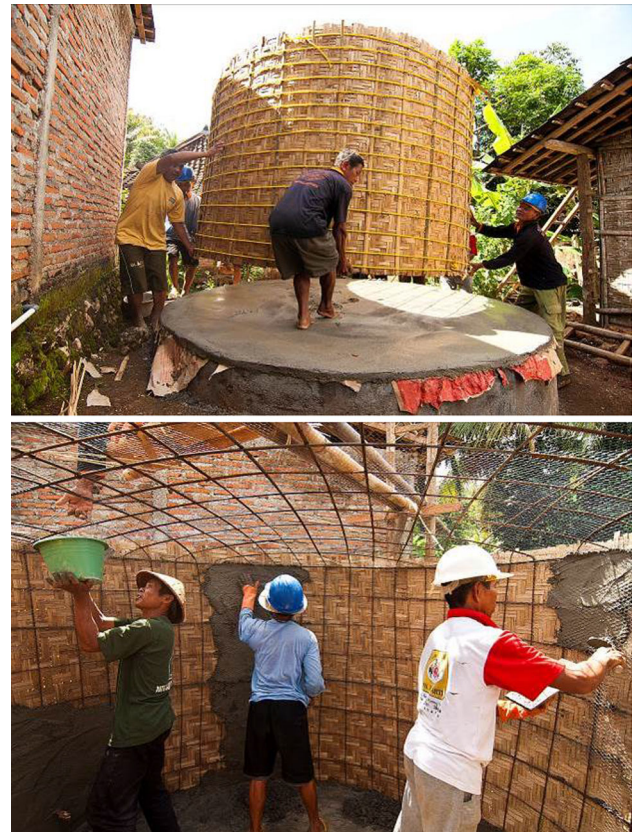
Fig. 3 Transport of the prefabricated reinforcement cage to the cistern foundation which has been treated with a screed on a decoupling layer of old cement bags before (top) and application of the inner mortar layer (bottom)
