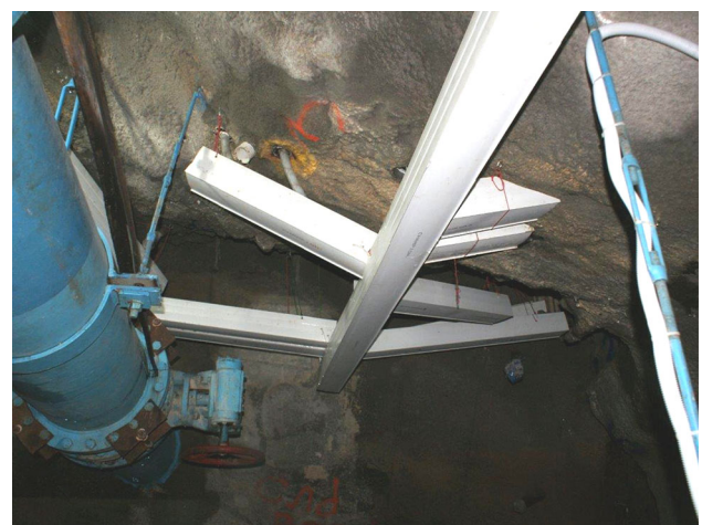
Fig. 14 Seepage water catchment for automated seepage monitoring
